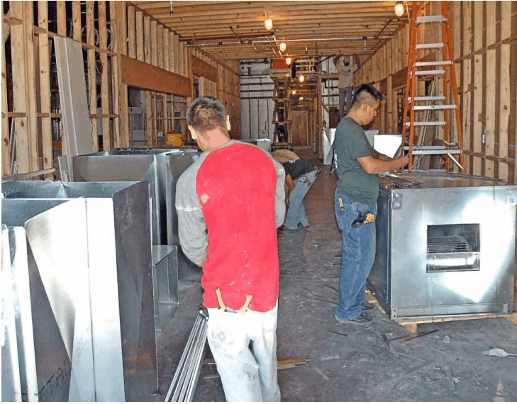
Large Air Conditioning and Heating ducts are being prepared for installation in the Fellowship Hall Ceiling (photos at left and below)
